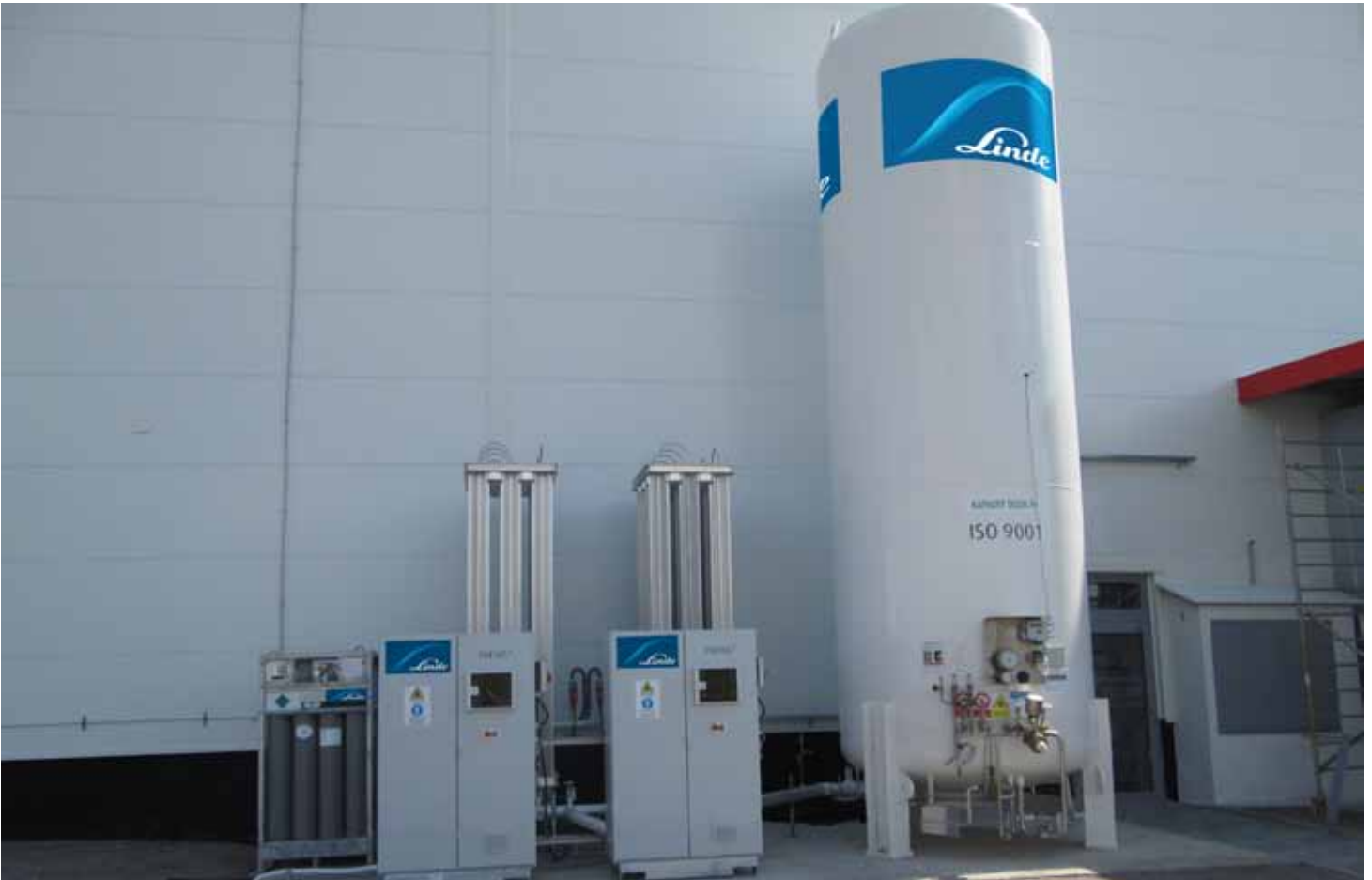
The centrepiece of the PLASTINUM® Gas Injection Moulding technology in Ostrov: the PRESUS® N10 pressure booster, which is supplied with liquid nitrogen from a tank. (Source: Linde)
