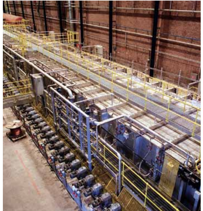
Roller hearth heating furnace with REBOX® oxyfuel solution including ceramic oxyfuel burners and Linde control system
