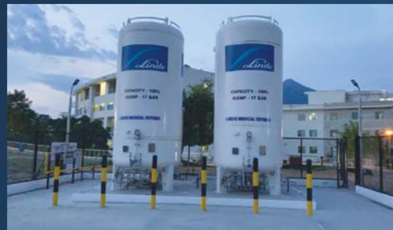
Linde India's installation at Shri Mata Vaishno Devi Narayana Super-Speciality Hospital, Katra, Jammu.
