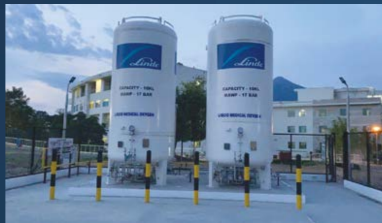
Linde India's installation at Shri Mata Vaishno Devi Narayana Super-Speciality Hospital, Katra, Jammu.
