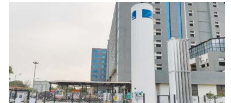
Medical oxygen installation at various partner hospitals to ease the supply of oxygen. Among others, Linde recently installed a 20 KL tank at GMERS Medical College, Junagadh, Gujarat.
