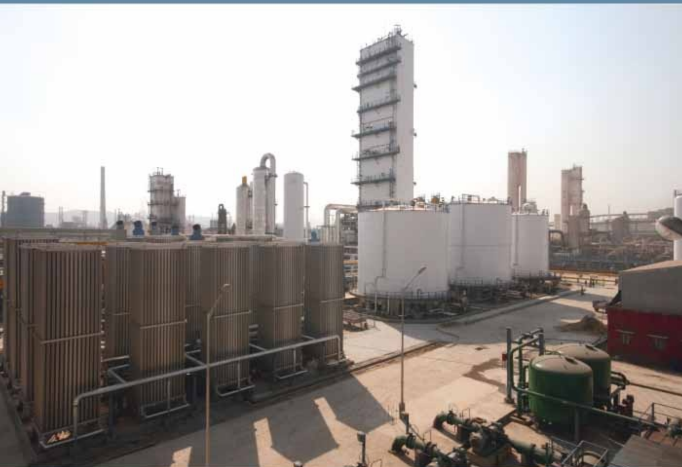
A view of the 1800 tpd plant at Bellary
