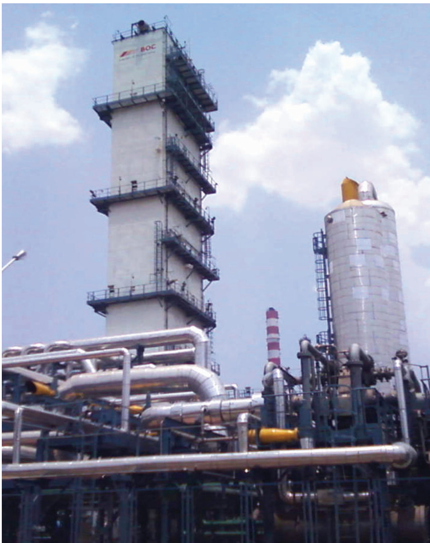
The state of the art, 1800 tpd Air Separation Unit at JSW Steel Works at Bellary, a testimony to BOC India's partnership with the steel major
